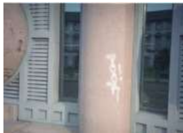
Pillar/Pillar/Support+ Wall (Item: PooR!)
