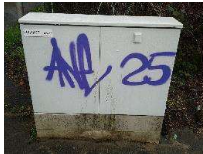
Power/distribution box (Item: ANe 25)
